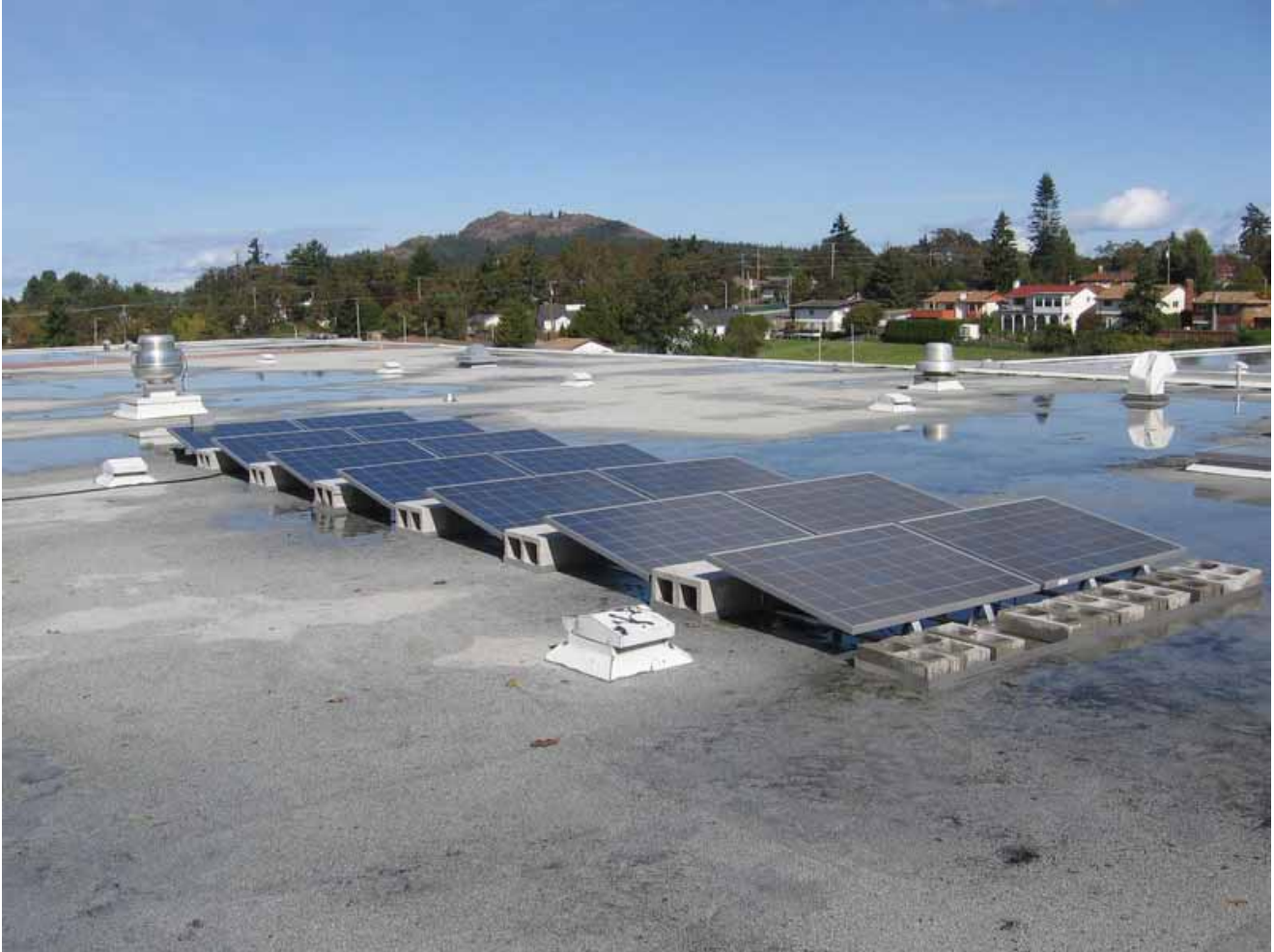
Figure 1: Rooftop PV Array
