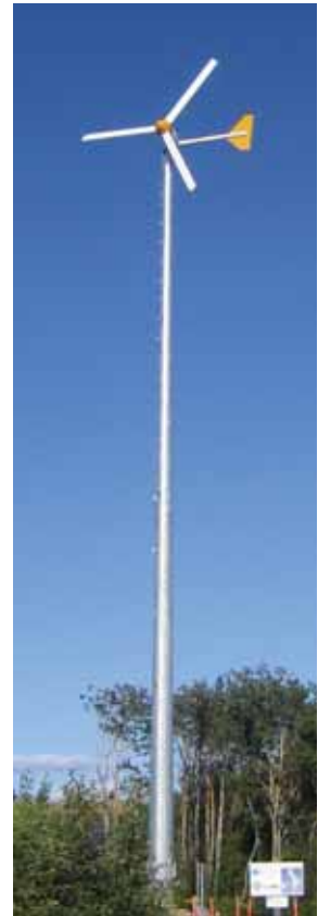
Figure 4: 10kW Bergey Wind Turbine
